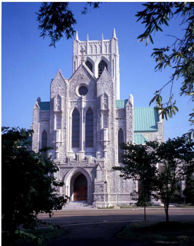
Prolific church architect William Halsey Wood designed St. Mary's Episcopal Cathedral in Memphis, a circa-1900 English Gothic marvel carved from limestone. Hord Architects re-roofed the structure and cleaned and restored the masonry. Photo: Carter Hord
